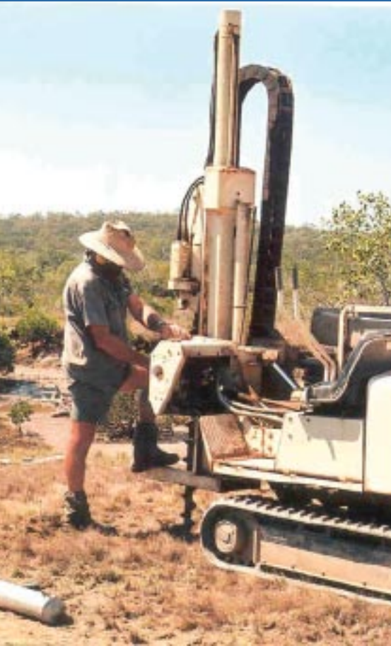
A drill used to install a piezometer in the acid sulfate soil study at The Narrows area, north of Gladstone
